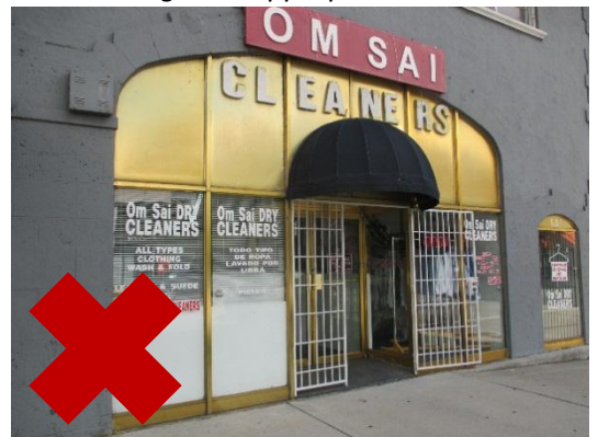
3.12 Awning is too small for opening
